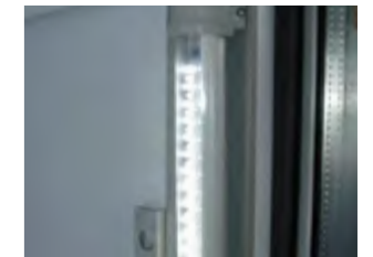
Illuminazione a led LED lighting
